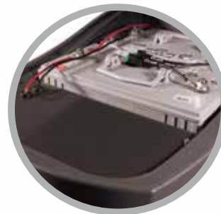
Maintenance-free, gel batteries are standard
